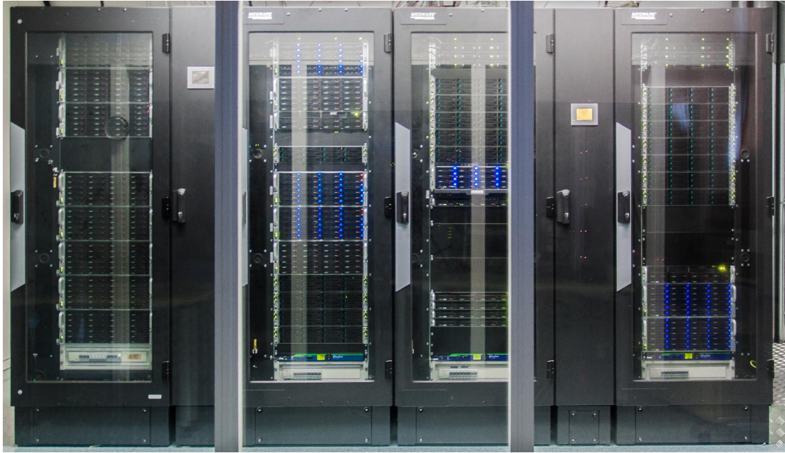
Figure 18: New computer cluster, January 2016 (photo H. Rottmann)
